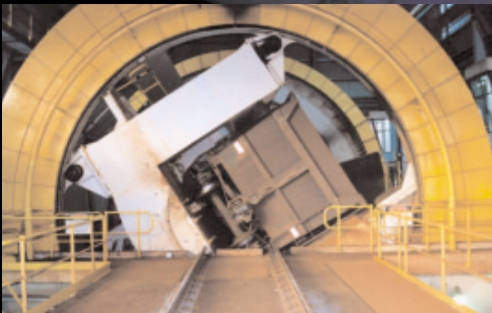
One of three rotary car dumpers used to offload ore at Port Hedland
