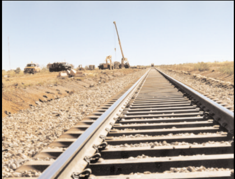
Steel Sleepered Track at BHP Iron Ore
